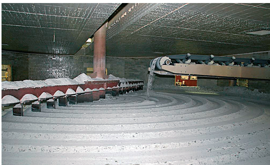
The Cameron Family Glass Packaging plant in the USA required a furnace of 254 tonnes/day capacity, almost double the size of its nearest Electroglass relative.
